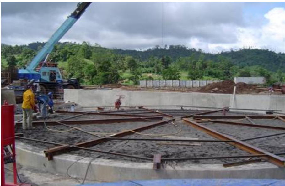
Figure 4: Footings for CIL plant leach tanks. Leach tank sections are on site and ready for assembly
